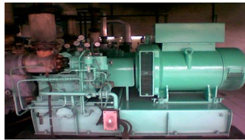
Gambar 1. Pengkopelan Turbin – Generator
