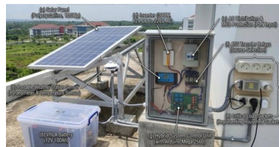
Figure 2. Experimental setup of the hybrid PLN–PV system installed at ITERA
