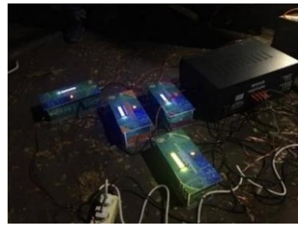
Figure 19. Active Noise Control Instrument
