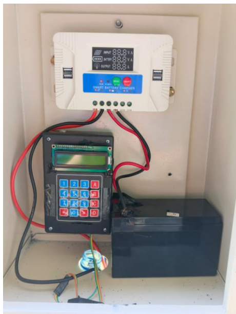
Figure 4. Implementation of electrical circuits and controllers
